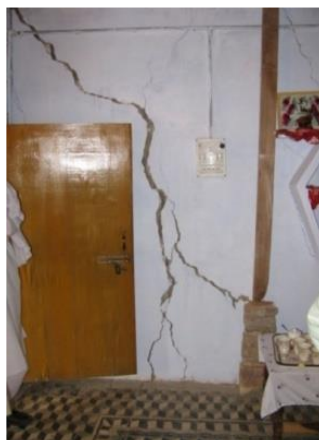
(b) Cracks near the door opening in the stone masonry
