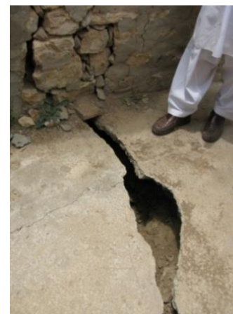
(c) Cracks in floor system
