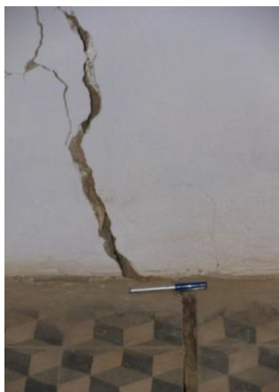
(a) Cracks in solid stone masonry wall
